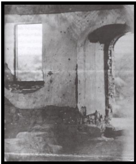
Interior View, no later than 1871. Note missing door, windows, window sashes, and floor. There is extensive water damage.
